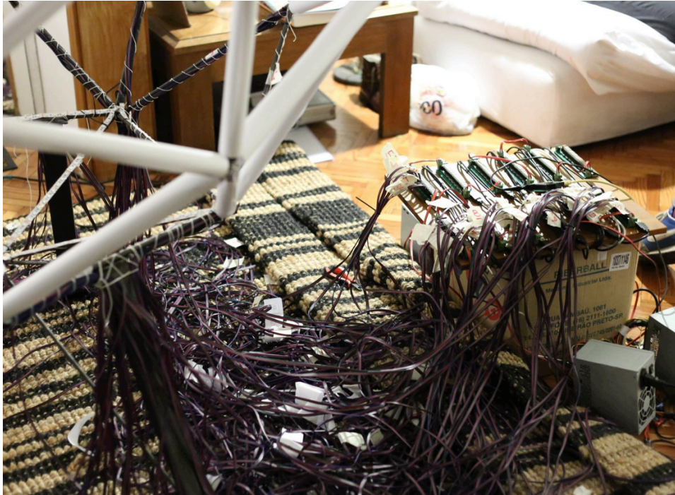
Figure 38 – Barcelona 's metallic structure, LED stripes, cables, LED drivers, and power sources.
