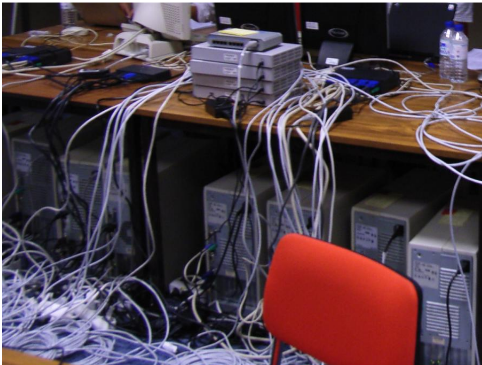
Figure 3.6: Cabling required for TAHI's solution deployment
